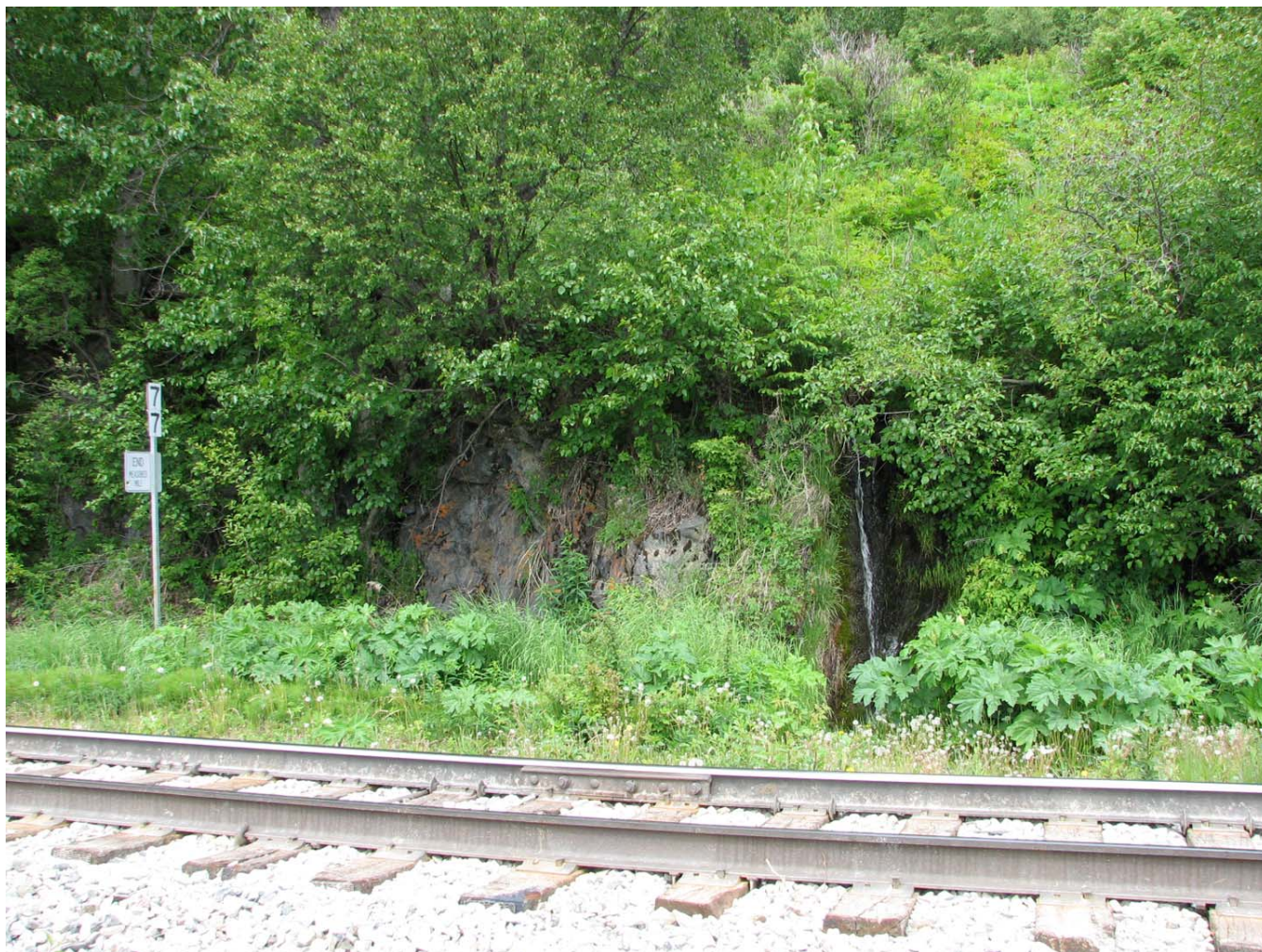
Fig 5. MP 77 and one of a dozen waterfalls in this stretch that are clearly within 100' of the track (photo by C. Northon on 6/12/10)
