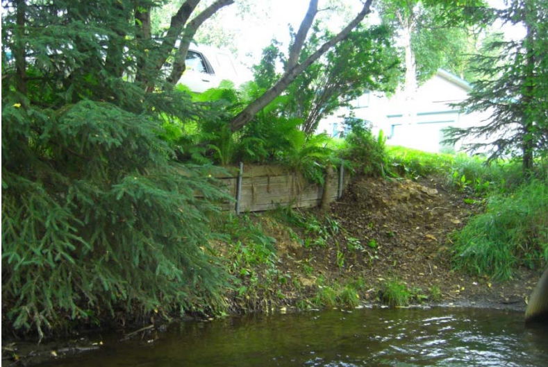
Figure B-3 – One of the many trails leading down to the water's edge. Many of the trails leading to the water were devoid of vegetation, allowing for more fines to find their way into the water.
