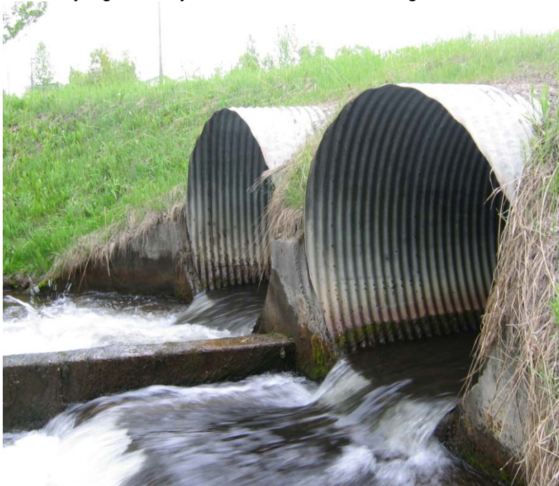
Figure B-2 – The culverts taking the water under Lake Otis Parkway to Hillstrand Pond. Note the extremely high velocity in which the water is exiting the culverts.
